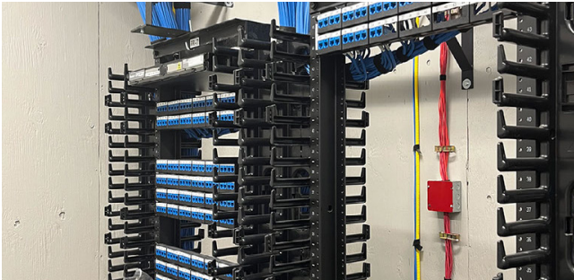
Second Floor Data Room
